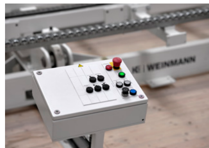
Local control panel With complete control system.
